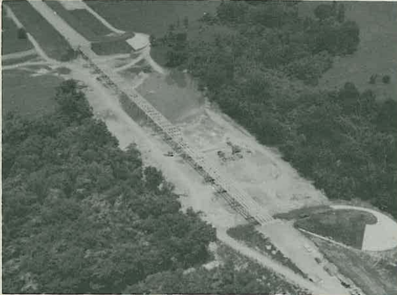
The East relief opening is 1,000 feet long, with pre-stressed girders in place for all spans.
