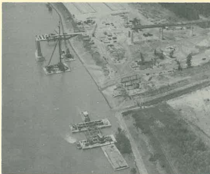
Here are piers No. 10 and No. 11, and part of the West approach to the main river bridge.
